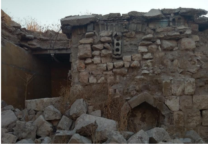
Damaged room façade, east of the courtyard (Museum for Islamic Art-Berlin, September 2019)
