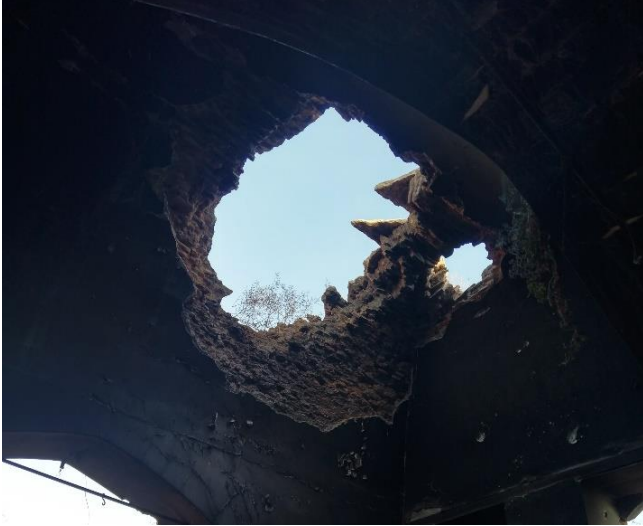
Damaged vault, western the prayer hall (Museum for Islamic Art-Berlin, September, 2019)
