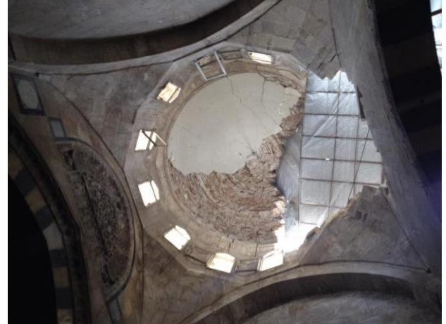
The damage of the dome Saleh Zakkour, Facebook page (April 22, 2017)
