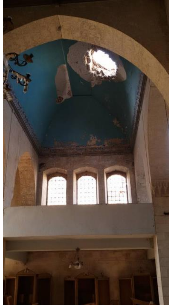
Damaged vault inside the Syriac Catholic Church
