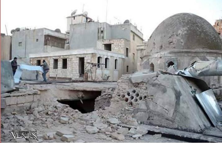
The damage at the roof of the church, APSA (January 9, 2015)
