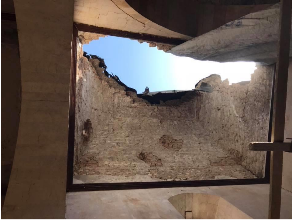
Greek Orthodox Church, a damaged vault of the church roof
